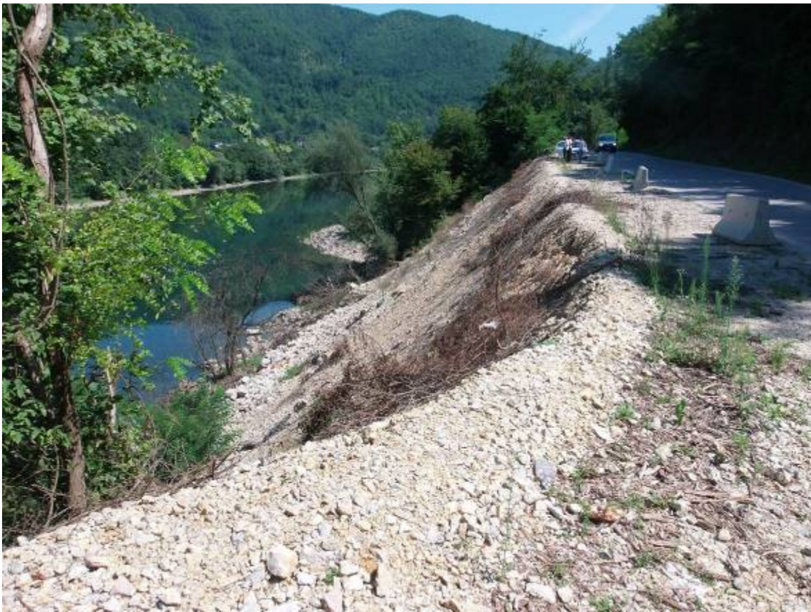
Picture 37. Landslide from km 6+000 to km 6+200
