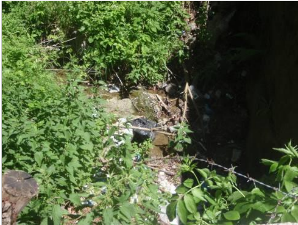
Picture 13 - Culvert covered with vegetation and waste
