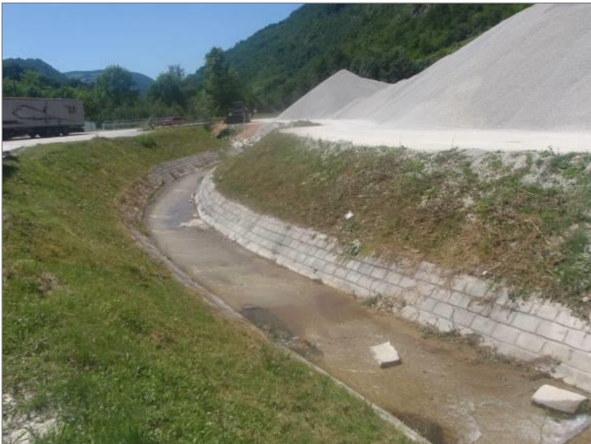
Picture 7 - Regulated river bed of Kozlica river in the area of the quarry
