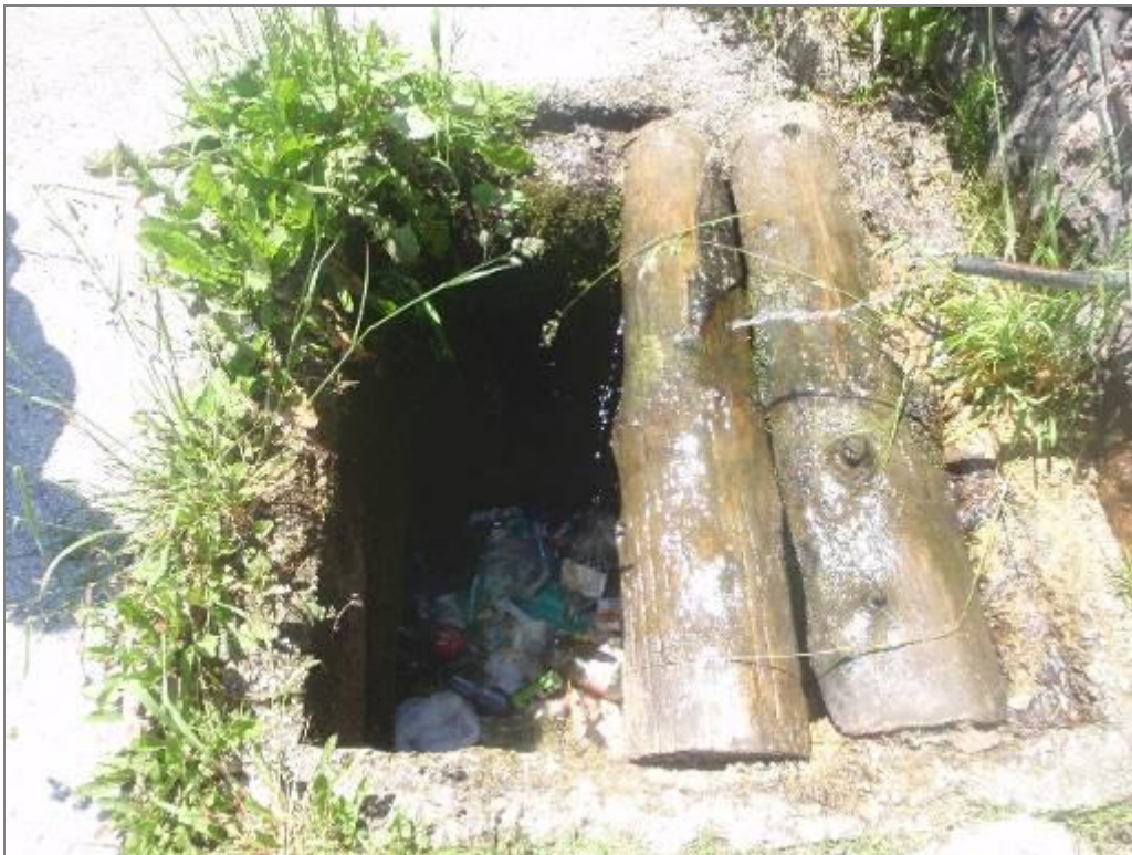
Picture 16 - Garbage in the drain
