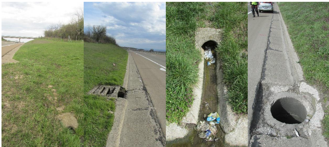
Figure 10. Gutters on the subject section
