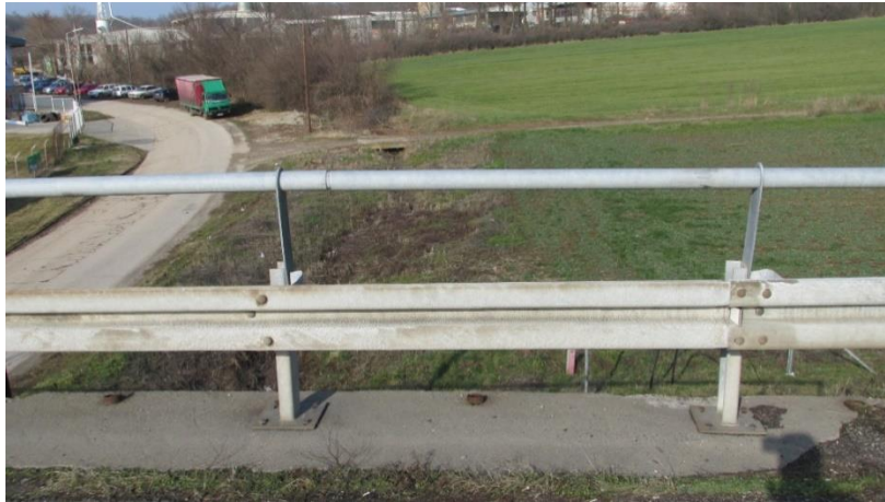
Figure 14. The Bridge over an unregulated stream and road of lower class at km 373+165
