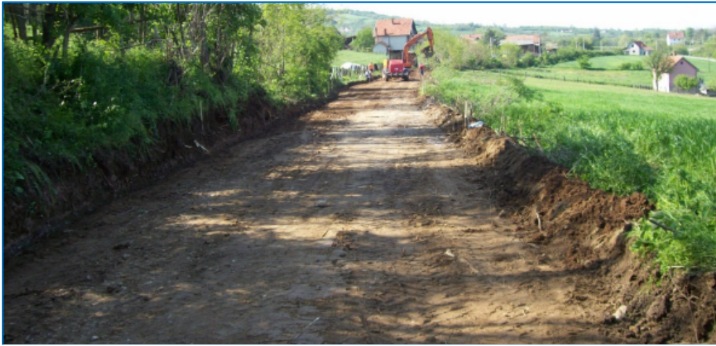
Photograph 7. Construction of a local road in the village of Stepanje, Lajkovac Municipality (Photo by V. Popadic)
