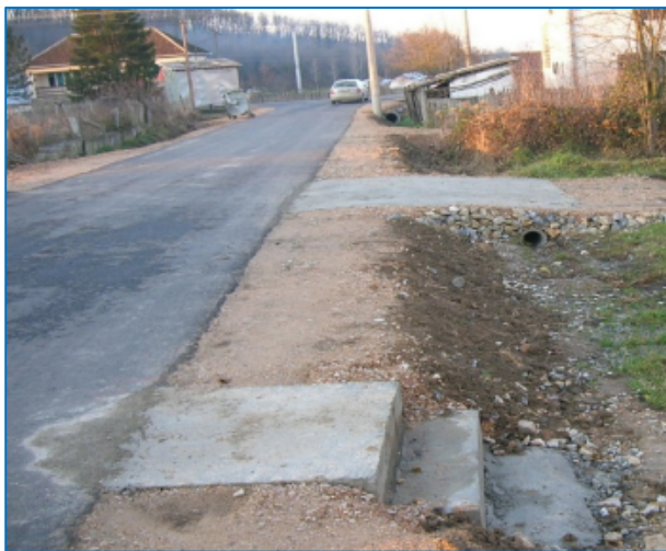
Photograph 10. Construction of a local road in the village of Vravec, Lajkovac Municipality
