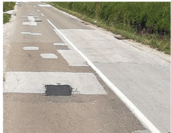
Photograph 10. Detail of pavement damage construction of the local road (Photo: V. Popadic)
