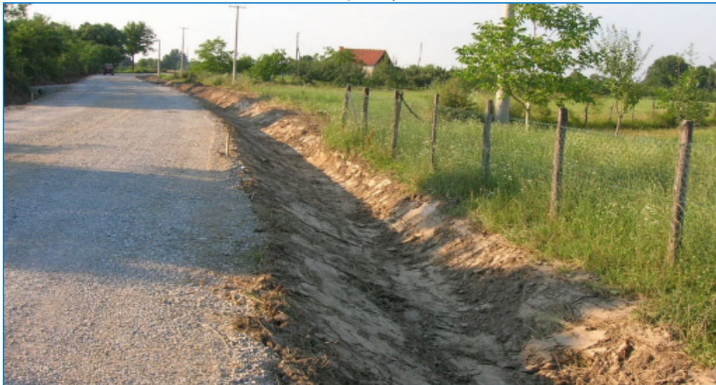
Photograph 9. Construction of a local road in the village of Vravec, Lajkovac Municipality (Photo by V. Popadic)
