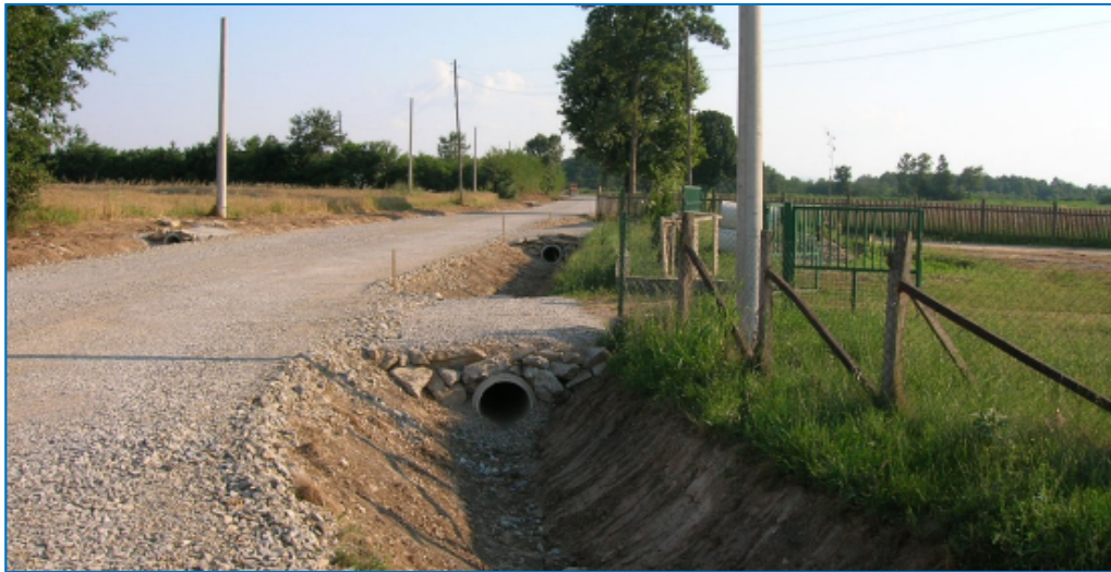
Photograph 8. Construction of a local road in the village of Vravec, Lajkovac Municipality (Photo by V. Popadic)
