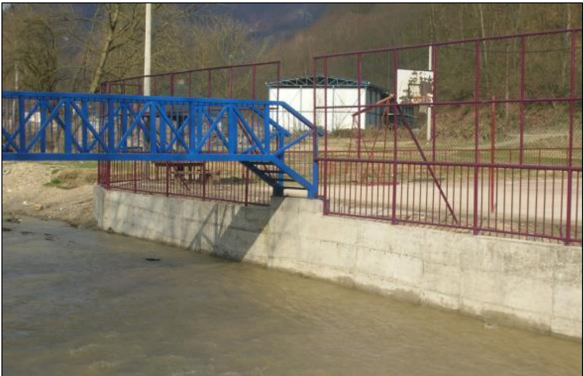
Picture 19. Pedestrian bridge, downstream from the bridge on the river Velika Reka
