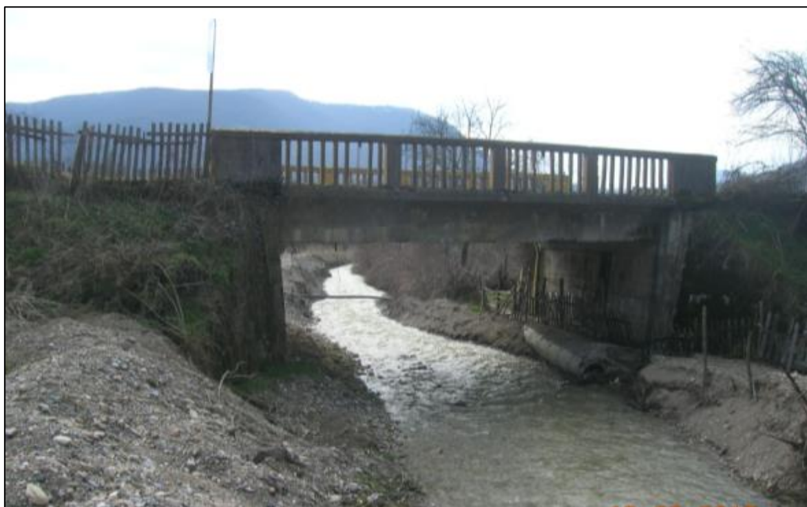
Picture 17. Upstream face of the bridge on the river Culinska Reka ~ km 18+000
